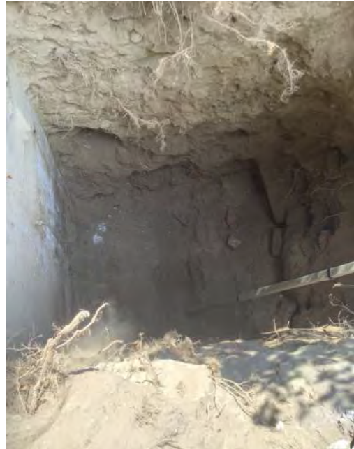
Photograph No. 6: View of 2050 Mass Ave foundation adjacent to obstruction.
