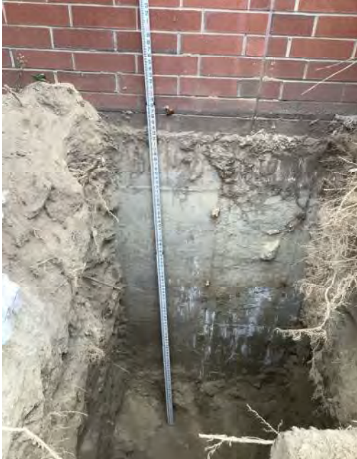
Photograph No. 4: View facing 2050 Mass Ave foundation wall. Rod positioned on top of foundation.
