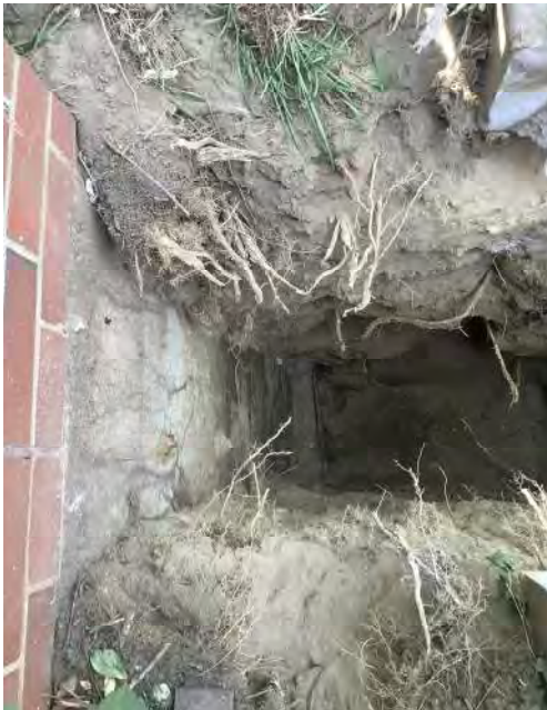
Photograph No. 3: View facing southwestern corner of 2050 Mass Ave building. Existing foundation appears to protrude 6 in. from face of wall.
